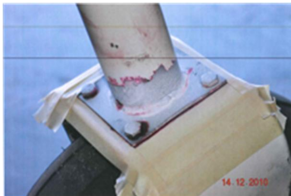
Photo 2: Cracking on the NLG leg and plate weld
